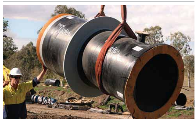
Flange joint Steel fittings
